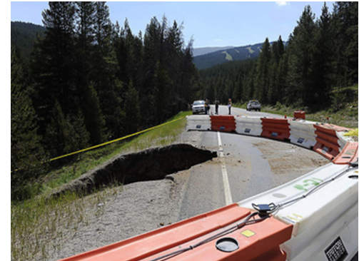
Figure 1. Example of culvert failure (Source: FHWA)
