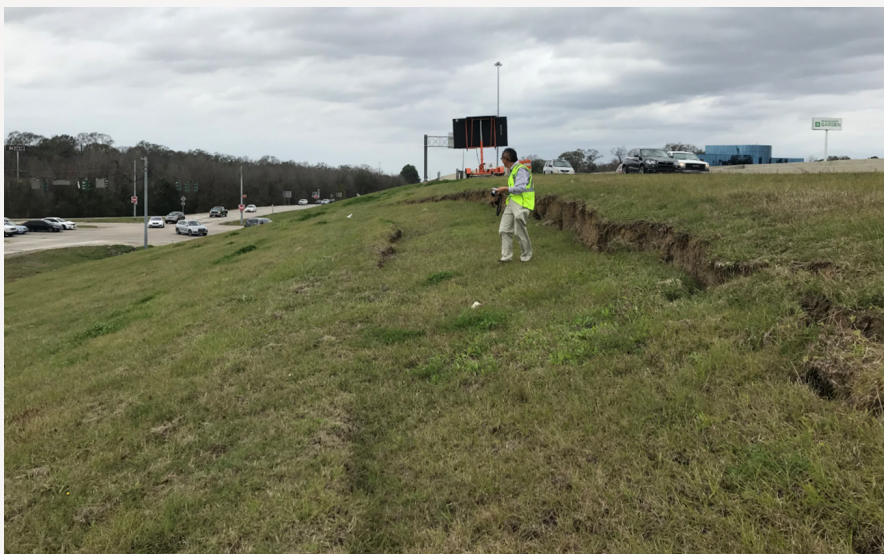
Figure 2. Slope failure on I-10 near Bluebonnet Blvd in Baton Rouge, LA (2019)
