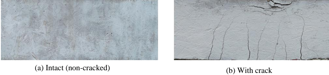
Figure 4. Illustration of intact and cracked concrete beams from experiments
