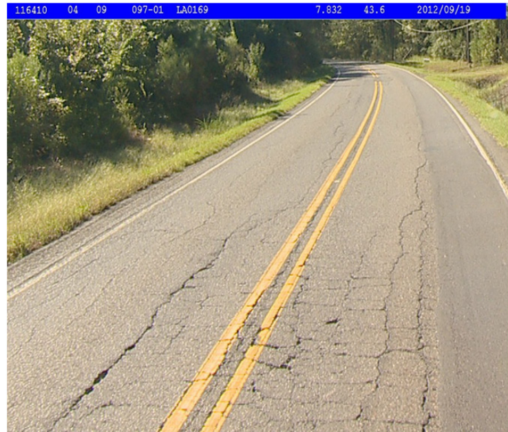
A damaged section of LA 169
